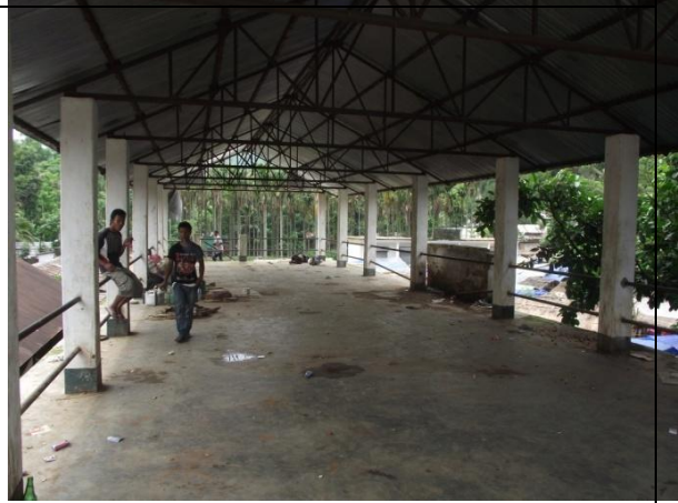
Upper floor of market shed not used as access is via stairs
